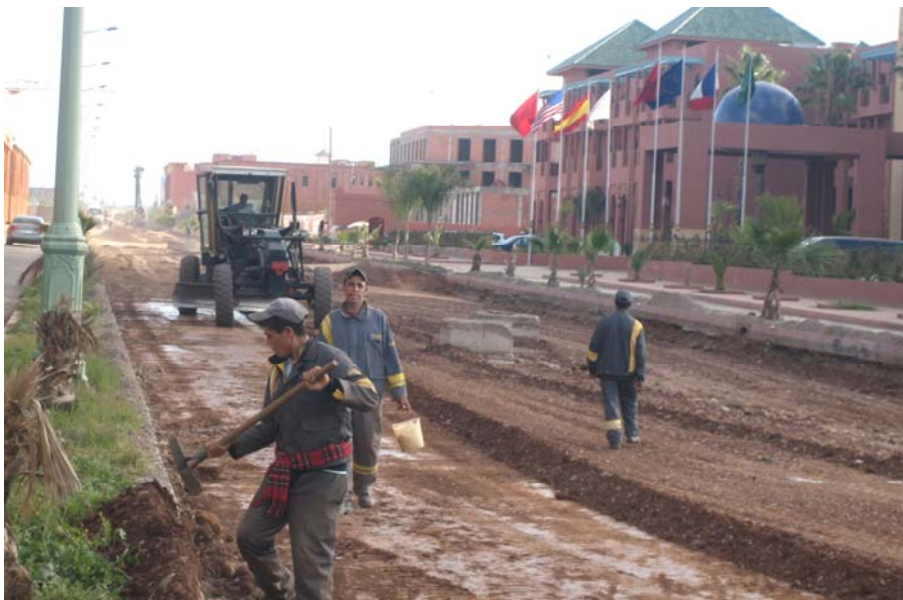
Works progress in Marrakech in view of the WTCC Race of Morocco
